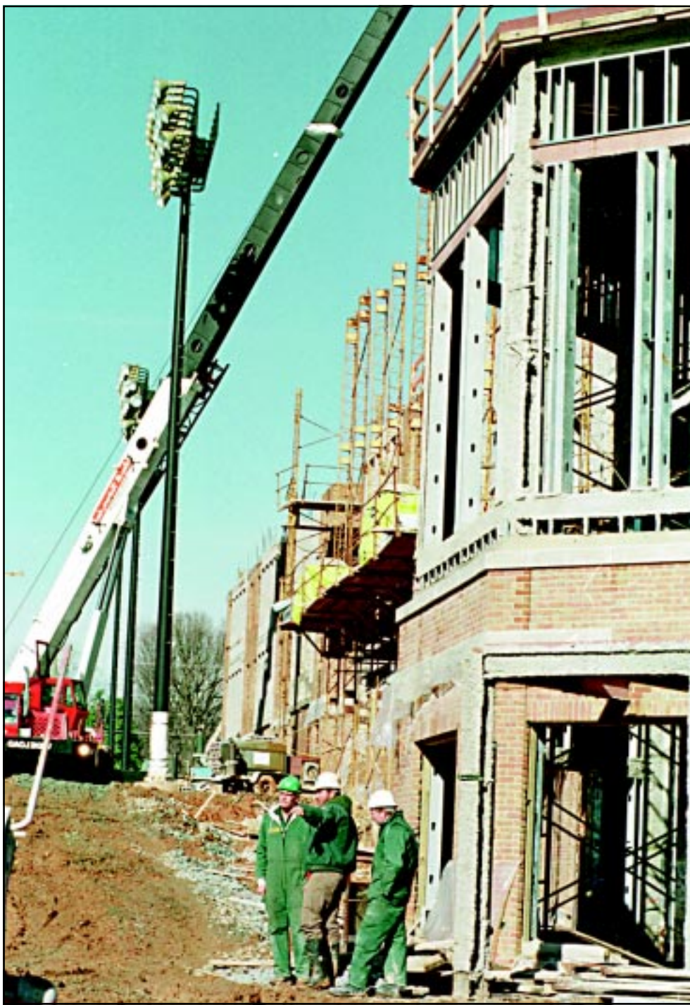
Construction workers confer next to the new residence hall, currently known as Polo Residence Hall. The building is part of the Board of Trustees' plan to create a residence for independent students.
